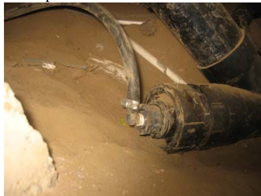
View of the water treatment system attached directly to the sewer line
