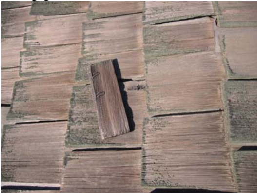
Sample view of damaged roofing materials
