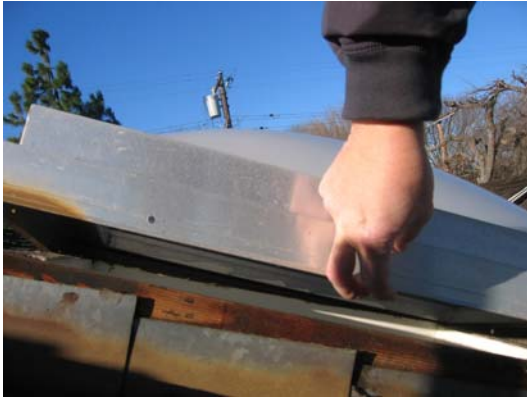
Sample view of a loose non anchored skylight
