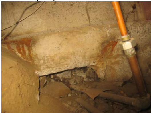
View of the soils subsided under the foundation
