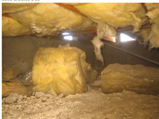
Sample view of fallen floor insulation under the master bedroom
