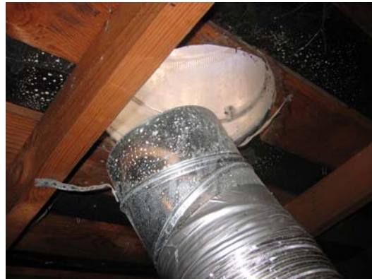
View of the kitchen exhaust duct not extended into the roof jack
