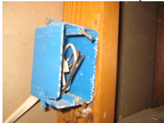
View of the exposed wiring at the master bath tub area
