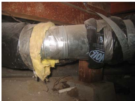
Sample view of ducting partially missing insulation
