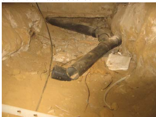
Sample view of building debris in the crawlspace
