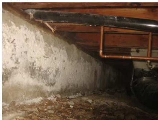
Sample view of efflorescence indicating water intrusion into the crawlspace
