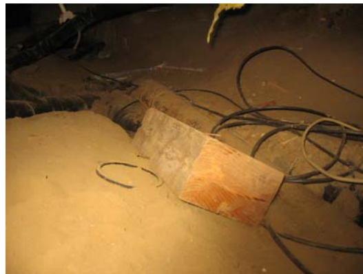
Sample view of wood debris in the crawlspace
