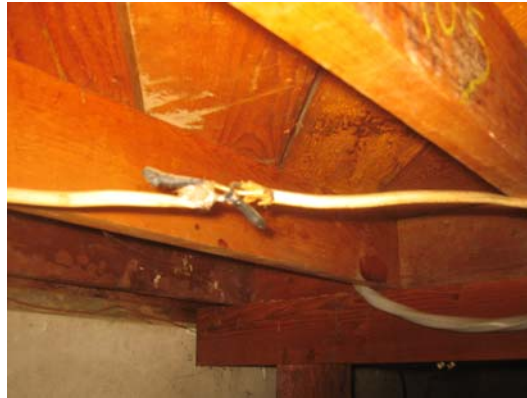
View of the spliced wiring not installed into a junction box under the rear right bedroom
